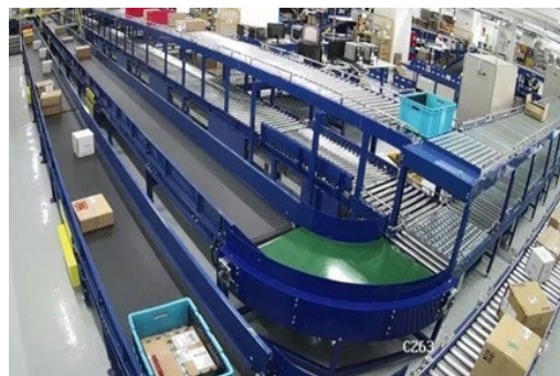
Outbound Conveyor Line
